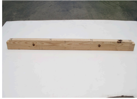
(2) Center Floor Joist with Notches
