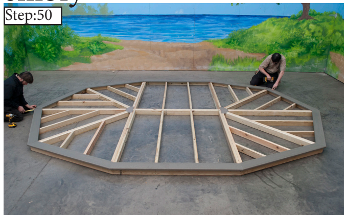
Step:50 Work your way around the perimeter and install all remaining Deck Boards.
