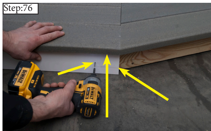
Step:76 Make flush with the corner of the Band Board and up against the Deck Boards. Fasten with 1 5/8" White Screws through pre-drilled holes.
