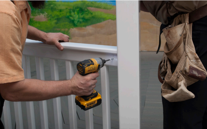
Fasten T Rail to Railing Inserts on the inside and outside using one (1) 1" Pan Head Screw through pre-drilled holes.
