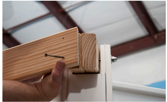
If the Roof Band Board is Short on the opposite side push up on the 2x4 Double Rafter as shown on next step.
