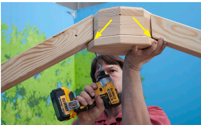
Pull Rafters down against the lip on the Compression Ring. Attach Rafters to Compression Ring from the bottom up using two (2) 3" Screws per Rafter.
