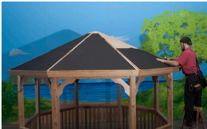
Install the Tar Paper on each Roof Section, as shown in previous steps.
