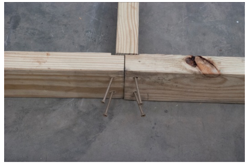
(21) Screw the rest of the band-boards into floor joists. Important! Band board splice needs to be tight.
