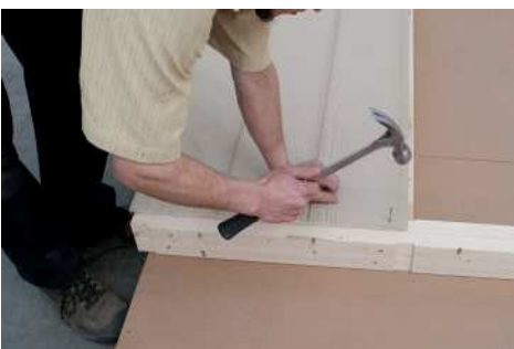
(47) Nail along the top, after making sure the siding is flush with the center of the double top plate as shown. Use an 8" to 12" nail spacing.
