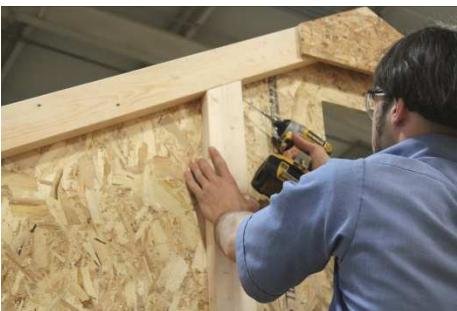
(128) Locate the 4 gable braces then fasten them at the siding splices in the peak, using 3" screws.
