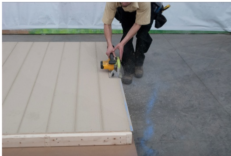
(56) Set the saw to 1/2" and cut along the line so that it is flush with wall frame, as shown in next step.
