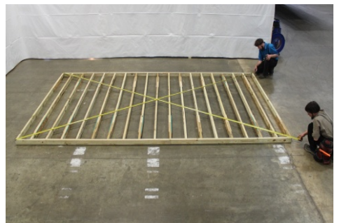
(24) Before proceeding, ensure that floor is square. Both measurements need to be equal. If Not: Knock the joists on the end accordingly, till measurements are equal.
