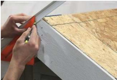
(188) Make a mark on the drip edge, parallel with the gable splice.
