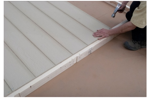
(52) Nail along the top, after making sure the siding is flush with the center of the double top plate.
