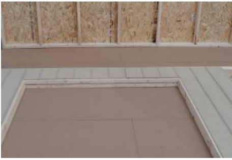
(86) Finish nailing the rest of the siding pieces on the front wall.
