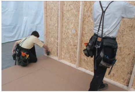
(69) Repeat for the rest of the wall, again; making sure wall is in against the floor frame.
