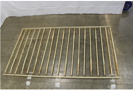
(16) Lay out the floor joists and band boards as shown, (12" on center) making sure to alternate the joist splices.
