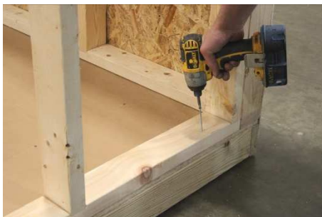
(92) Fasten the bottom plate to the floor, using 3" screws, every 12 to 14 inches, making sure the bottom plate is flush with the floor joist.
