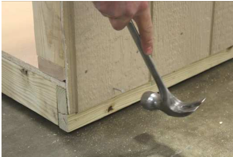
(71) Attach bottom edge of siding to floor, using an 8” to 12” nail spacing.
