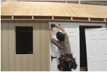
(167) Fasten the other hinges, keeping door flush with the trim on the left side.
