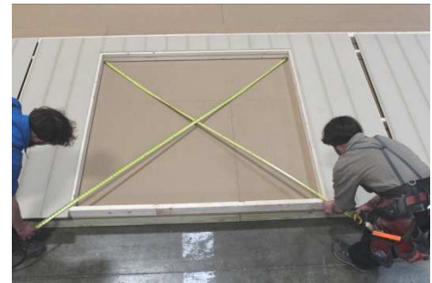
(85) Before completely fastening these pieces, check to see if the door opening is square. IF NOT, pull the bottom of the wall left or right to adjust it, then finish fastening these pieces.
