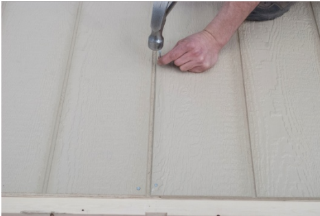
(53) Nail along the splice, making sure the splice is parallel, and looks similar to the other grooves.
