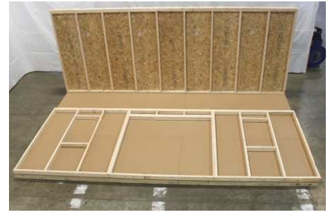
(79) Fasten the rest of the studs, using the same method as the back wall.
