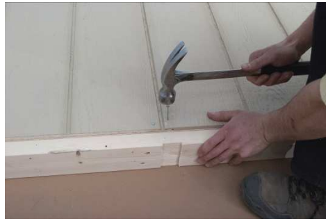
(51) Make sure the splice looks similar to the other grooves. Then fasten the corner of the siding to the plate.
