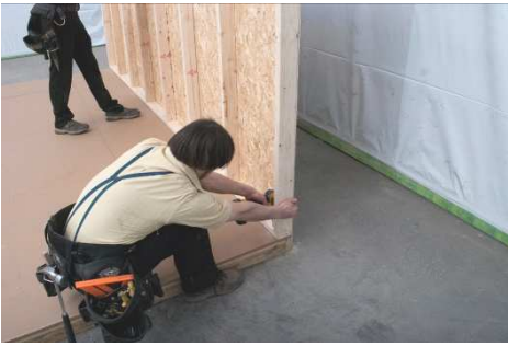
(68) Fasten to floor, using two 3” screws at every stud, trying to hit the floor joists.
