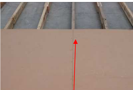
(31) Center the floor joist evenly with the flooring splice, then nail the corner, after making sure flooring is tight against, and flush with the previous piece. Nail this piece, using the same methods as the previous piece.
