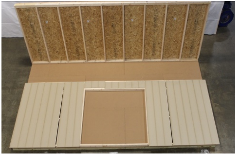
(80) Lay out siding as shown here, with the over lap towards the right. (Refer to drawings for door & window placements)
