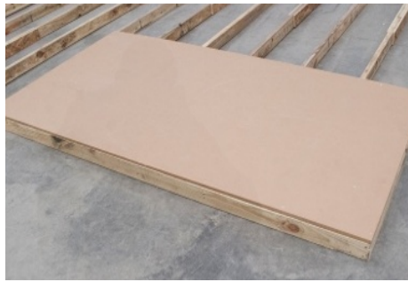
(29) Nail along the front side, again; making sure flooring is flush with the band board.
