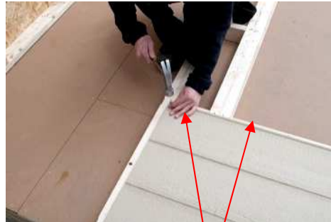
(81) Starting with the piece beside the door, place the siding even with the center of the double top plate, make sure siding has 3/4" reveal along edge of door frame, then nail along the top.
