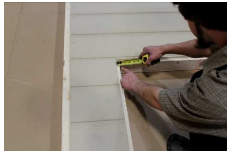
(84) Fasten the siding pieces above the doors, and keep it 3/4" above door header as shown; before nailing.
