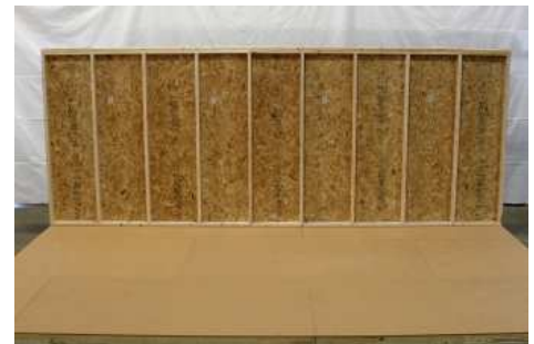
(73) Done! Make sure the wall is fastened securely before moving to front wall.
