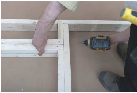
(77) Fasten both double door studs with dados, to the door header, using four 3" screws.
