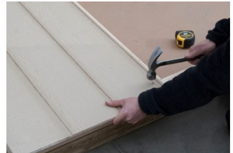
(82) Temporarily nail the bottom as shown, (Using only 1 Nail for now) and make sure siding has 3/4" reveal along edge of door frame.
