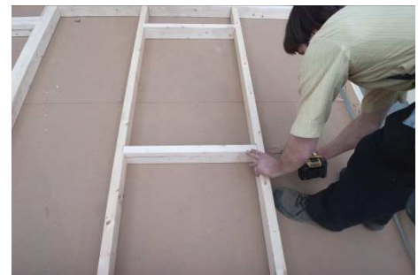
(76) Fasten window studs with dados, to the window blocks, using two 3” screws.
