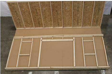
(74) Locate and lay out the parts to assemble the front wall. (Refer to drawings for door & window placements)
