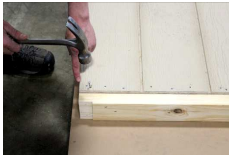
(45) Starting with the left piece, place the siding even with the center of the double top plate, and flush with the wall stud.
