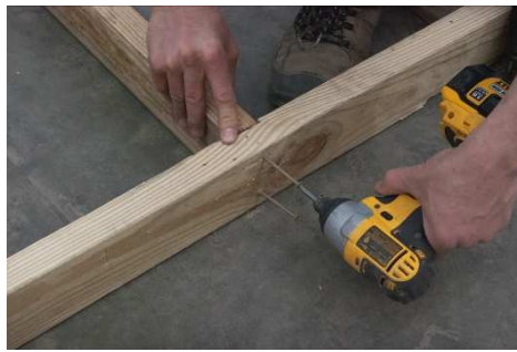
(20) Attach the rest of the band board, using 3" screws, through the pre-drilled holes.
