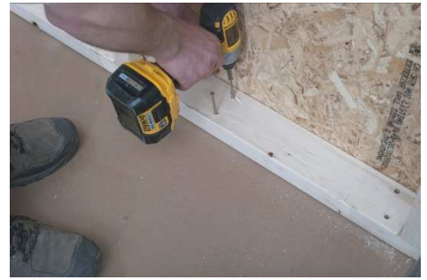
(70) Fasten the bottom wall plate at every floor joist, using two 3” screws.
